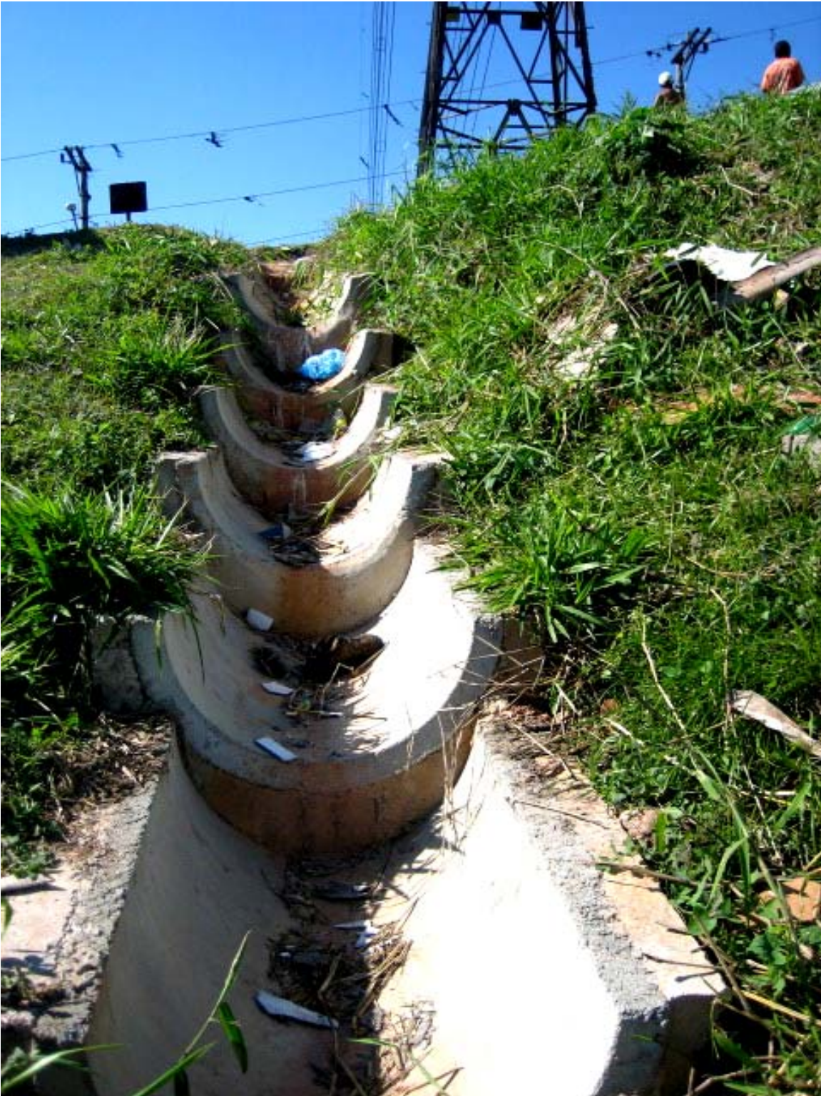
Storm water management system, installed by Petrobras engineers replaced open run off streams and reduces landslide
